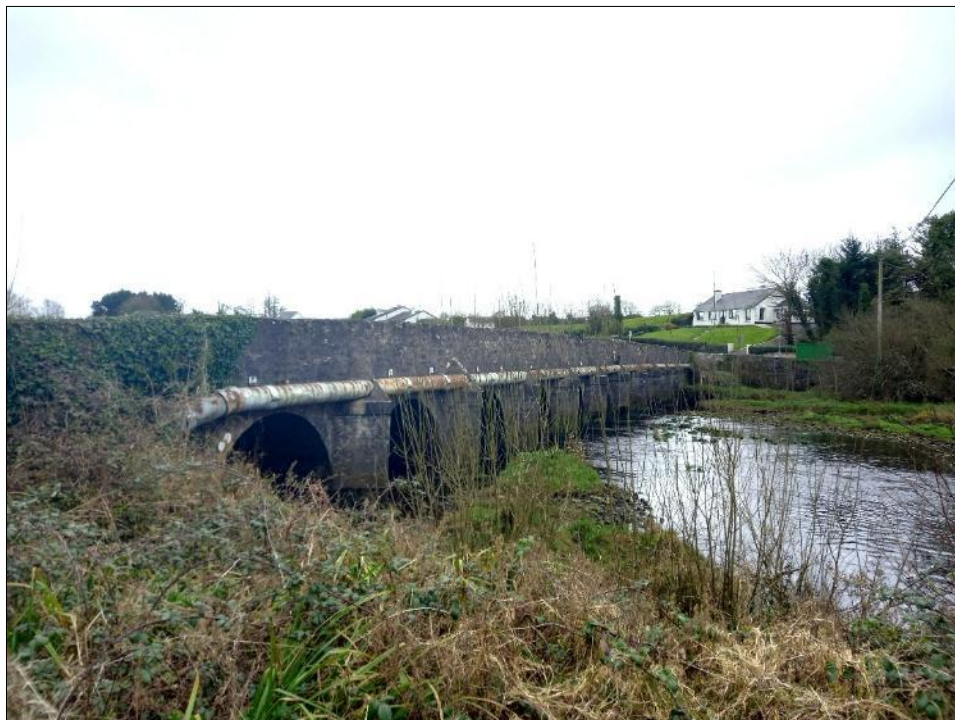
Plate 14.15: View of Palmerstown Bridge RPS 017, from northwest towards western elevation and utility piling sitting atop the bridge pier coping, along the full span of same
