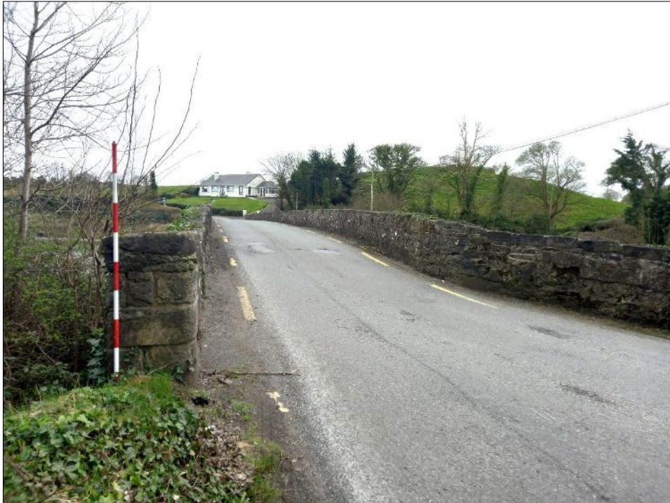
Plate 14.14: View of Palmerstown Bridge RPS 017, from north towards curved northeastern wing wall
